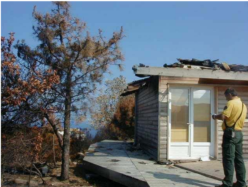
Figure 6b: Building partly destroyed by the Coti Chiavari wildfire
